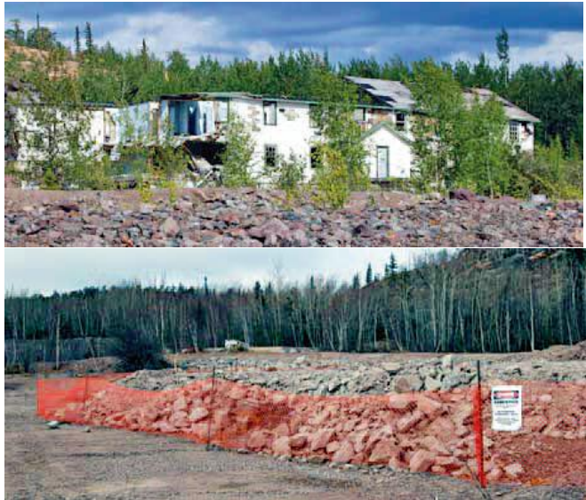
Example of “before” and “after” views of building demolition at the Gunnar site (2010).
