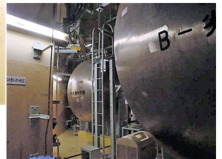
(劣化重水貯槽)
