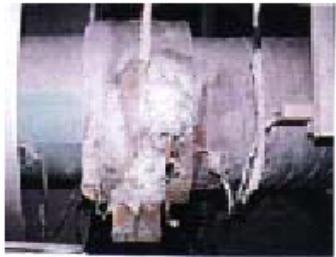
Condition around the broken temperature sensor
