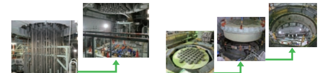
Dismantle and remove control rod guide tubes Removal of control rod drive unit support plug
