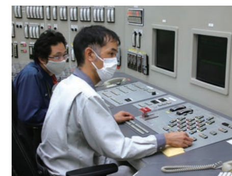
Control room at time of restart
