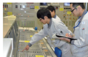
Control room for the Fuel Handling Facility
