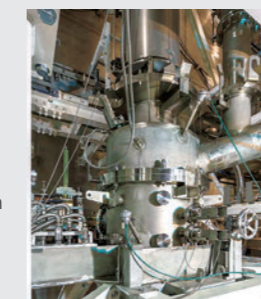
Incineration and Melting Equipment in OWTF
