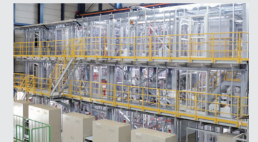
Continuous hydrogen production test facility made of industrial materials. H 2 production rate: 0.1 m 3 /h-H 2 Size: W18.5×D5×H 8.1 (m)
