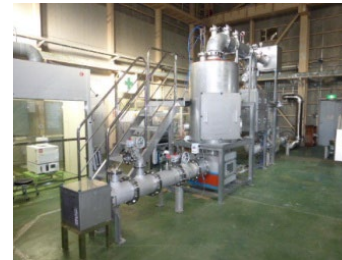
Apparatus for Evaluating Clogging Effect of HEPA Filter on Confinement Capability Under Fire Accident
